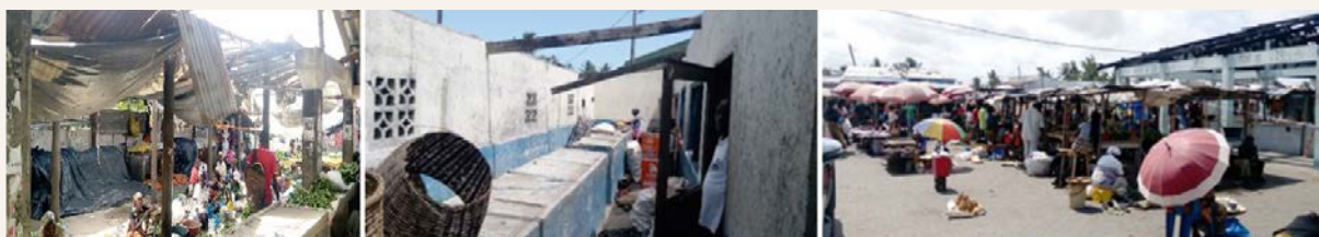
Figure 1: First two pictures on the left shows damaged roofs, and the third picture on the right Stalls empty and vendors selling their produce on the sidewalks after the market suffered cyclone damage.
